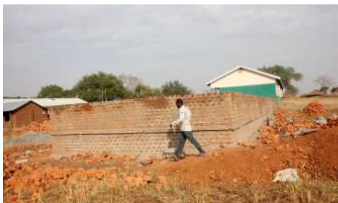
The super structure brick walls at window level coming up the superstructure walls completed; the timber roof structure also put in place. P1 teacher and Walter walking around appreciation of the new classroom
